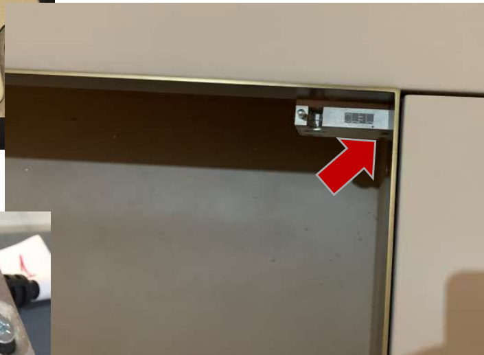
Top mounting give issues when door settle down.
