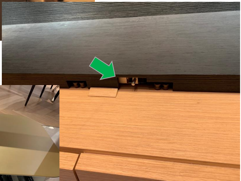
Lock well mounted
