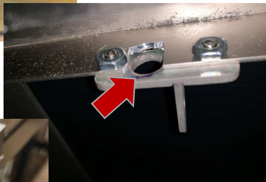
Sensor hole drilled gives constant alarms.
